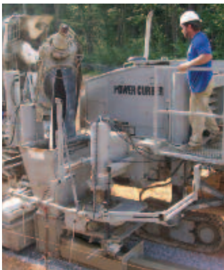
Operator has great visibility of entire process.
