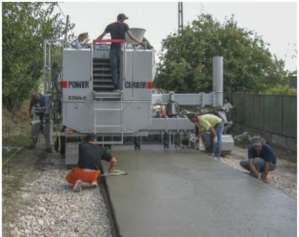
Paving 10' (3m) wide in Romania. Center pour paver is sectionalized for varying paving widths.
