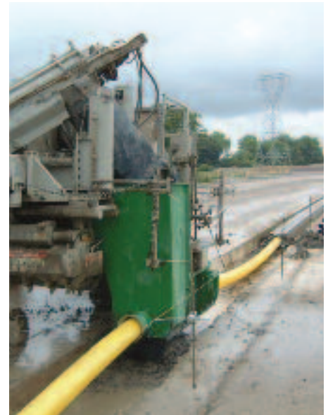
Slotted drain showing inflated tube.
