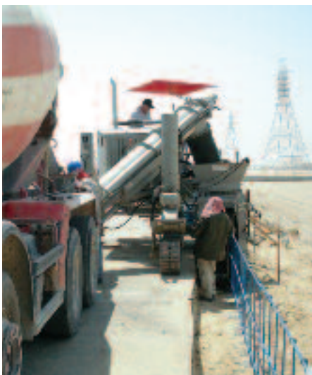
Barrier below grade with rebar.
