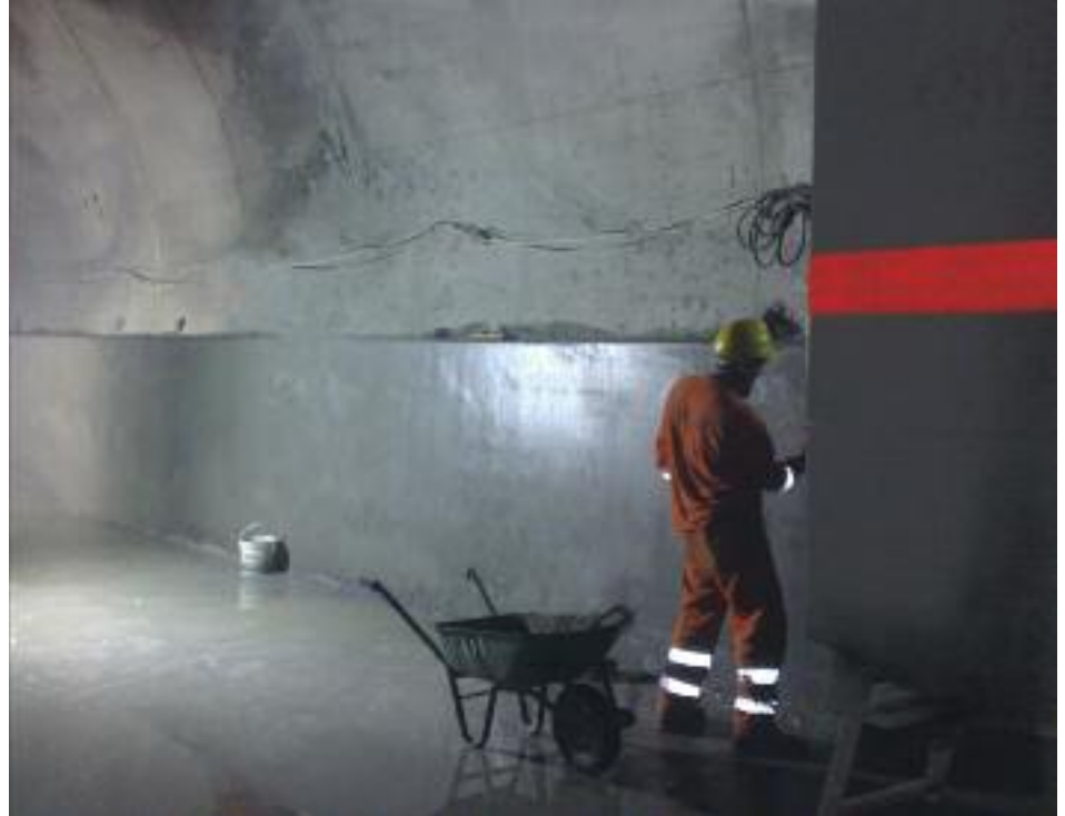
Platform & wall structure poured along a tunnel wall – mold is adjustable in height and width to accommodate varying tunnel diameter.
