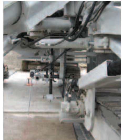
Parapet sensor mounting.
